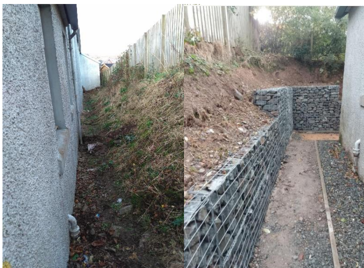
Image: Crossmichael Memorial Parish Hall before works to improve exterior (Left) and after (Right)
